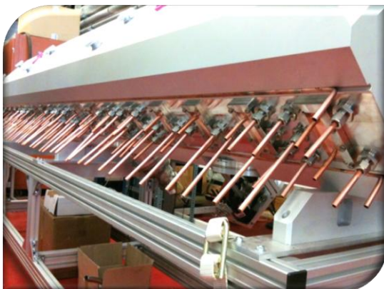
Cooling pipes with Swagelok fittings
